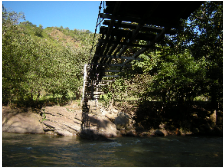
One by one, we crossed this damaged bridge during the trekking phrase
